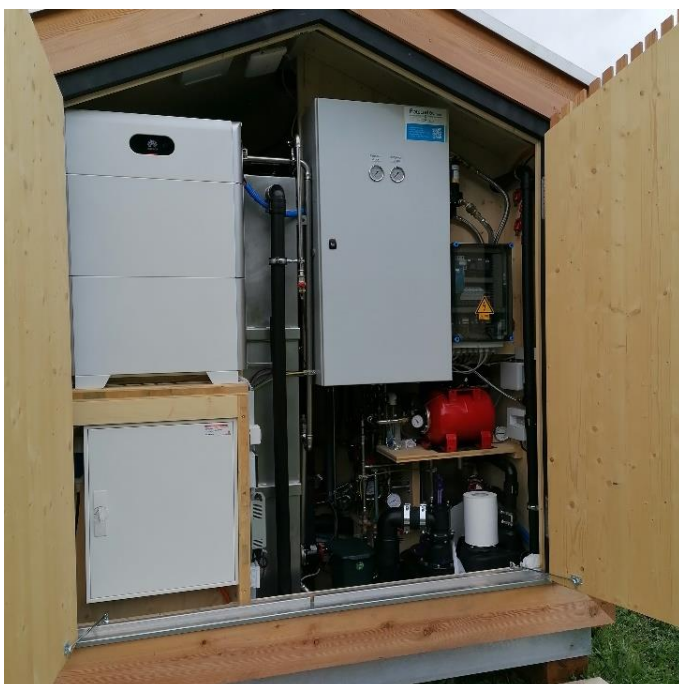
Wall mounting in the technic board
