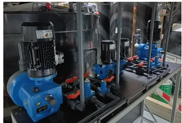
Detail Feed pumps
