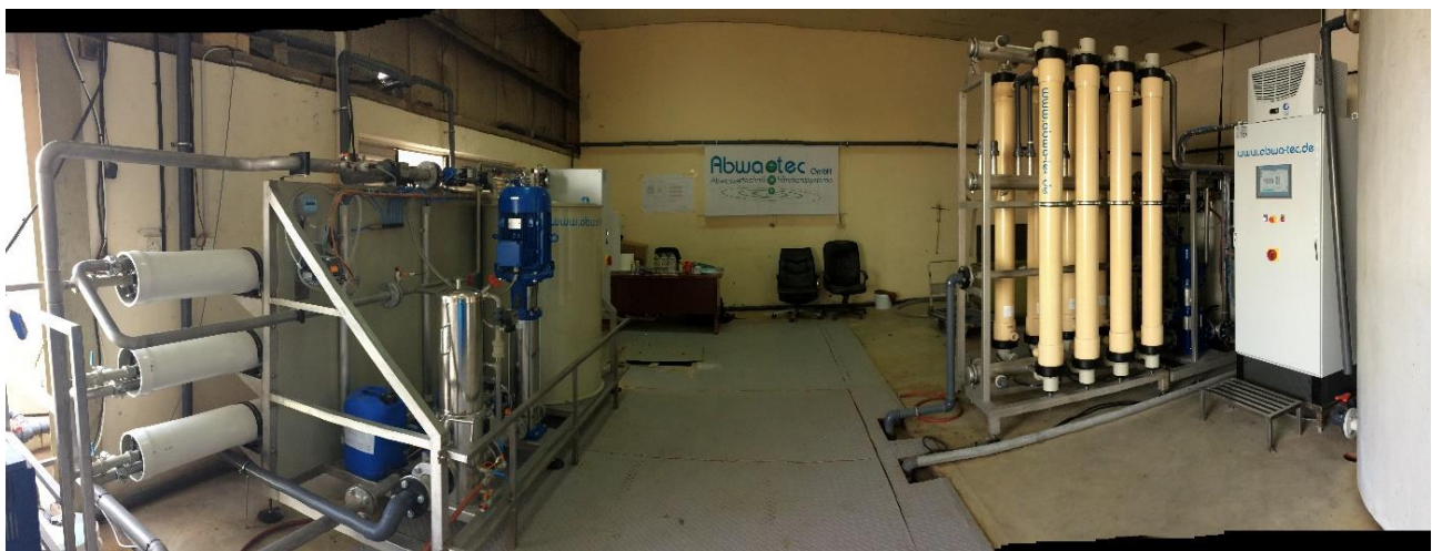
Plant overview – Reverse osmosis (left), Ultrafiltration (right)
