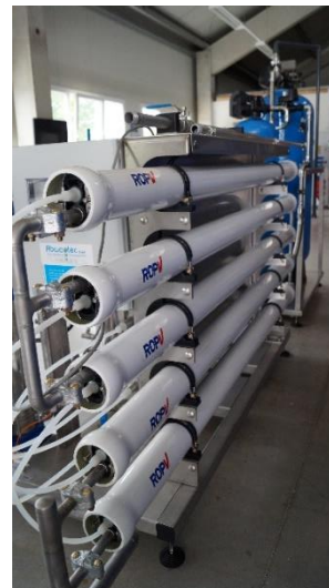
Detail reverse osmosis
