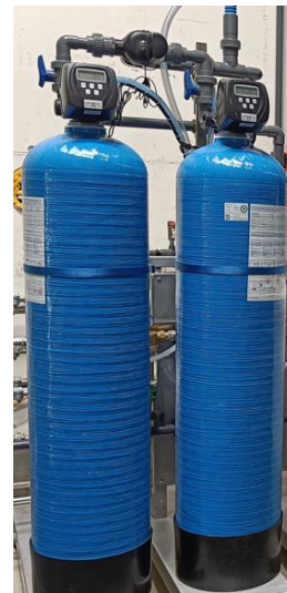
Double softening system
