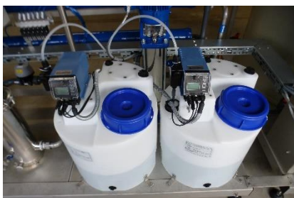
CIP-Station for chemical cleaning
